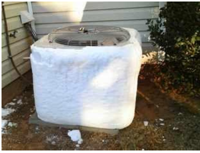
Figure 1. Too Much Frost for a Heat Pump.
